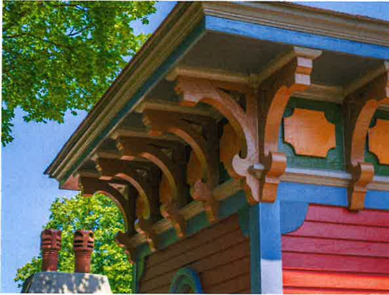
Left: Bracketed cornice and decorative frieze band under the eaves of the tower's hip roof.
